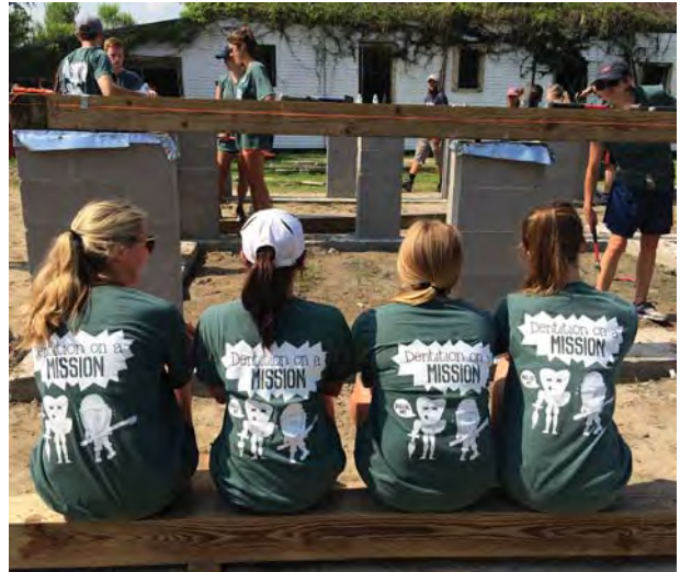
Incoming freshman and sophomore dental students braved the heat to build a house for Habitat for Humanity during the first LSUSD Root Camp: Detention on a Mission event.
